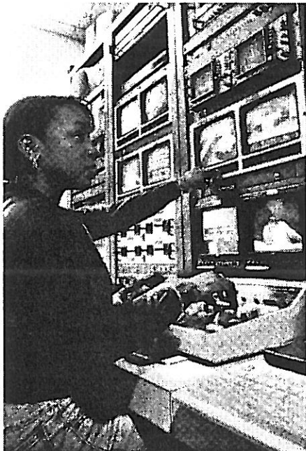
North Carolina Information Highway control room
